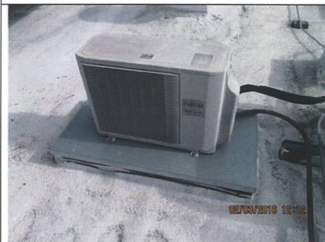
Item 40 condenser of projection booth AC unit – fair.
