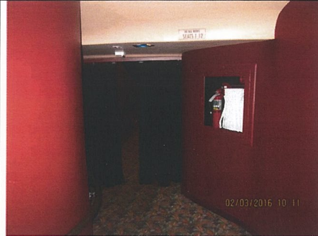
Item 44 fire hose cabinet. Fire hose system is served off the domestic water and not the new fire riser.
