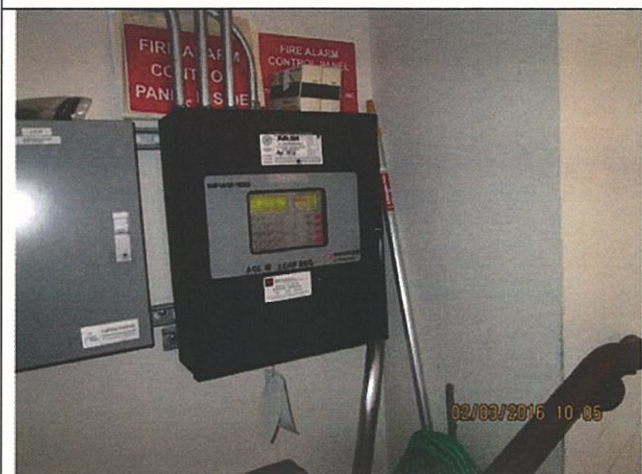
Item 42 Fire alarm system panel – good.
