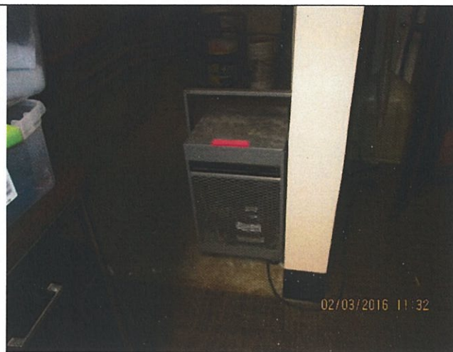
Item 46 Dehumidifier for area below stage – fair.
