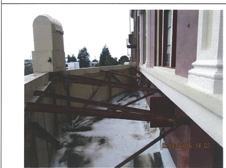
Item 5 Area above marquee – poor Comment: Paint is faded and steel supports are rusting. Exposure to salt laden fog accelerates deterioration.
