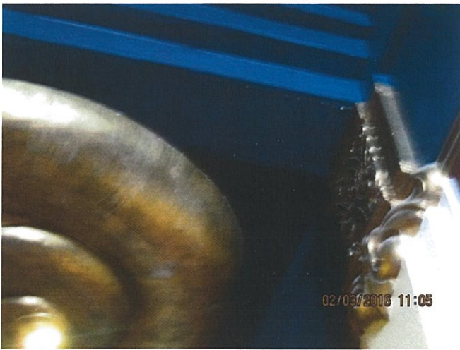
Item 17F: Crack at end of beam.
