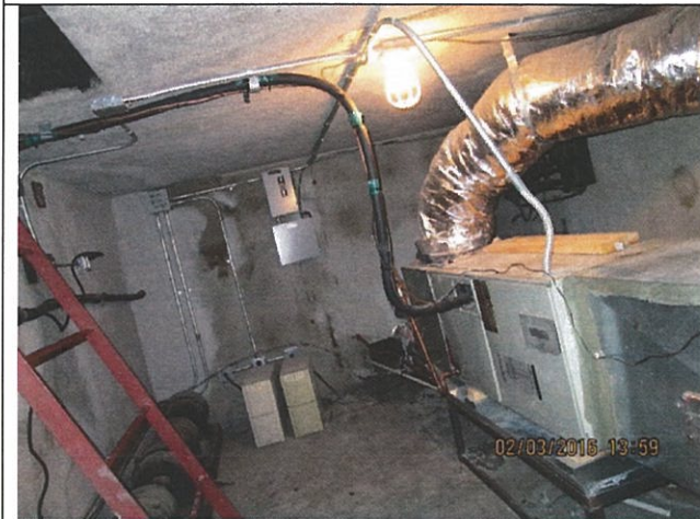
Item 39B evaporate for lobby split system - fair.
