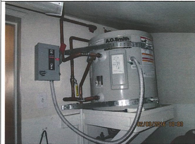
Item 41 19 gallon, 3000 watt, water heater – fair.
