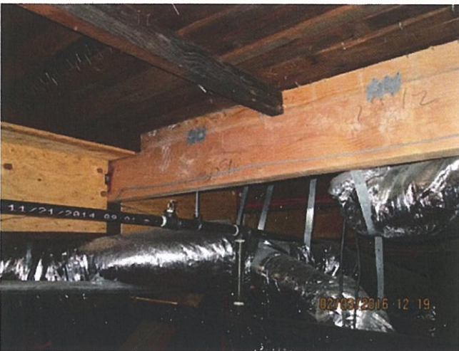
Item 36G: New exhaust vent ducts serving restrooms.
