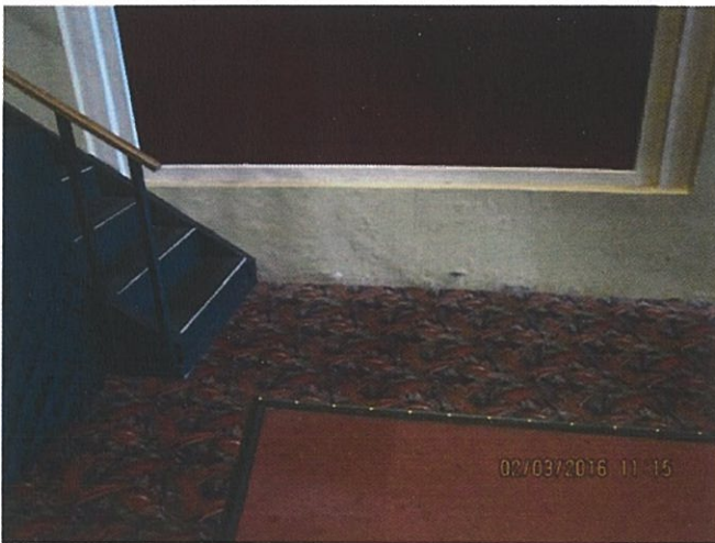
Item 17I: Minor paint peeling. This area appears to have repeated peeling. May be due to moisture behind wall, but none present on surface during walk.
