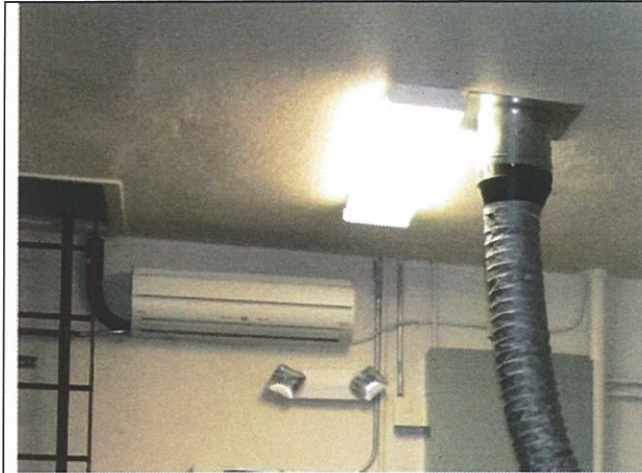
Item 40A evaporator for projection booth AC unit – fair.
