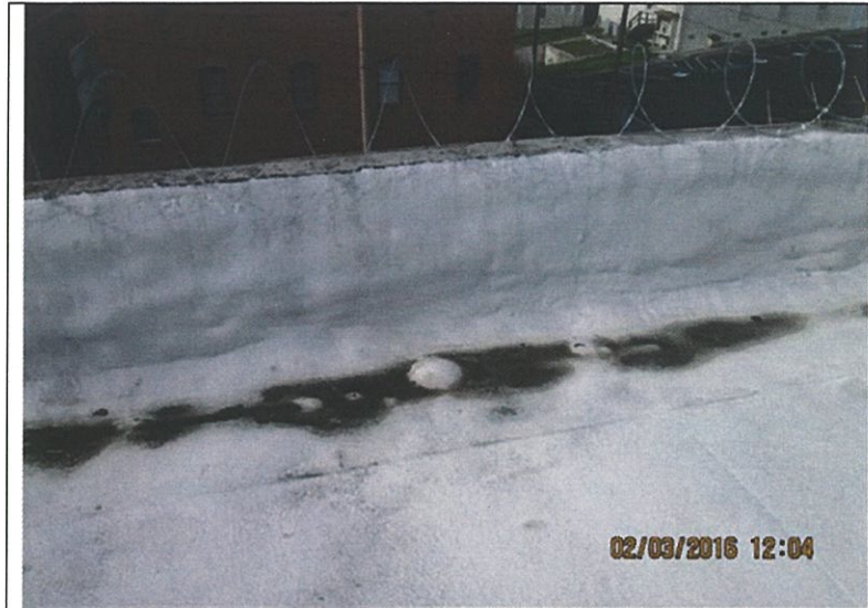
Item 8A Blisters in area of ponding water.
