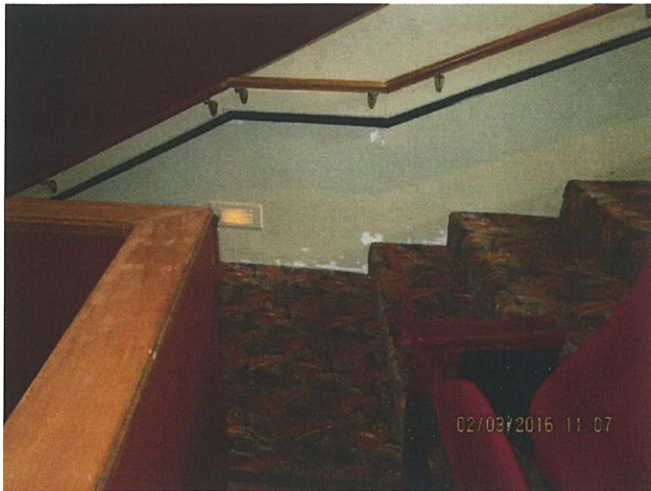
Item 17H: Minor paint peeling.
