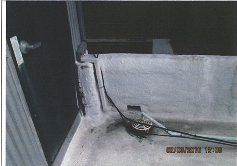
Item 8B Roof drains are clear at both sides of roof, but path to drains needs to be cleaned.
