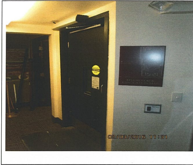
Item 47 passenger elevator (1 floor).
