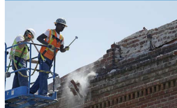
Workers clear damage from 2014 South Napa Earthquake. (Source: USA Today)
