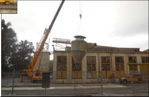
Building 106A Removal of Dangerous Conditions September 2014
