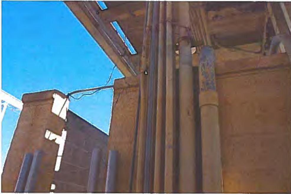
Image 10. West façade, the concrete wall cap and block are cracked.
