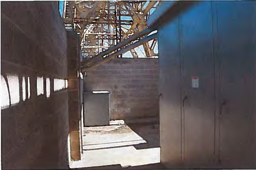
Image 12. Interior view looking east from the west entry. The concrete block walls and floor slab are unpainted. A large electrical vault is visible at the right.
