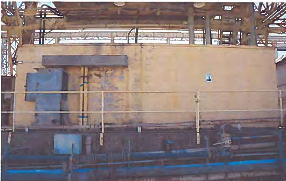
Image 6. North façade with miscellaneous electrical equipment at the east end. The lower part of the photo shows the wall of Building Ways #1 with large pipes running horizontally.
