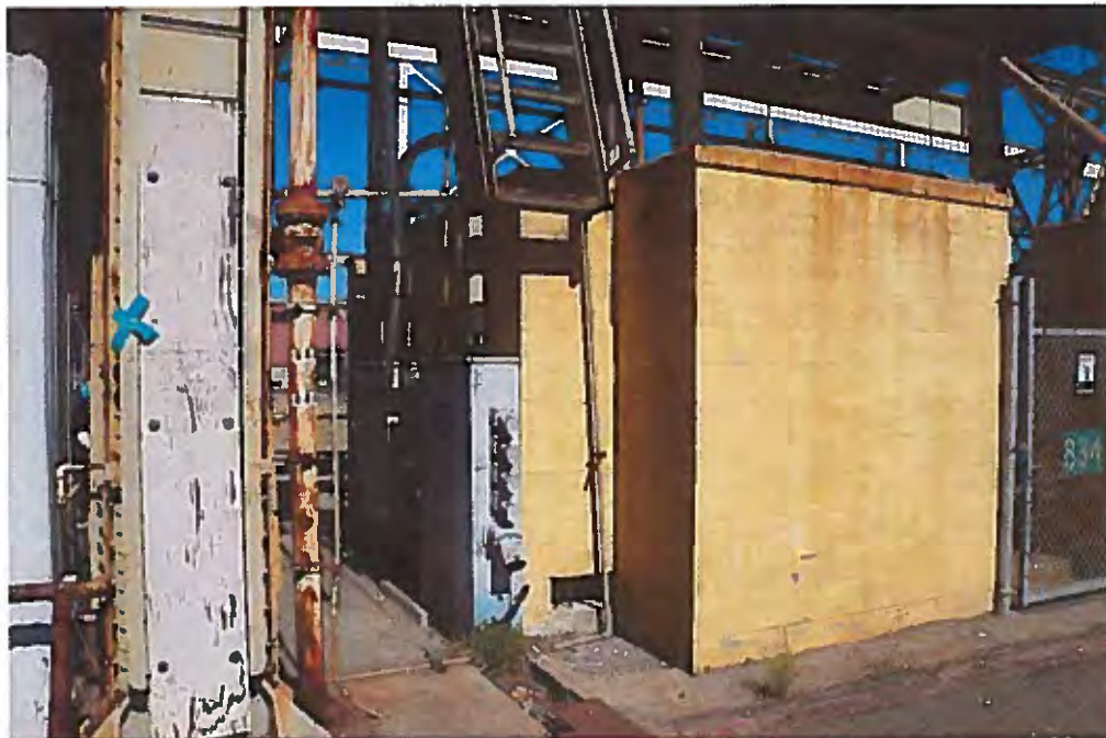
Image 4. South façade, west end. The west façade with electrical vaults is somewhat visible at the left.
