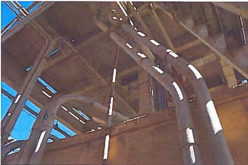
Image 16. Conduit extending to the gantry crane above Building 834.
