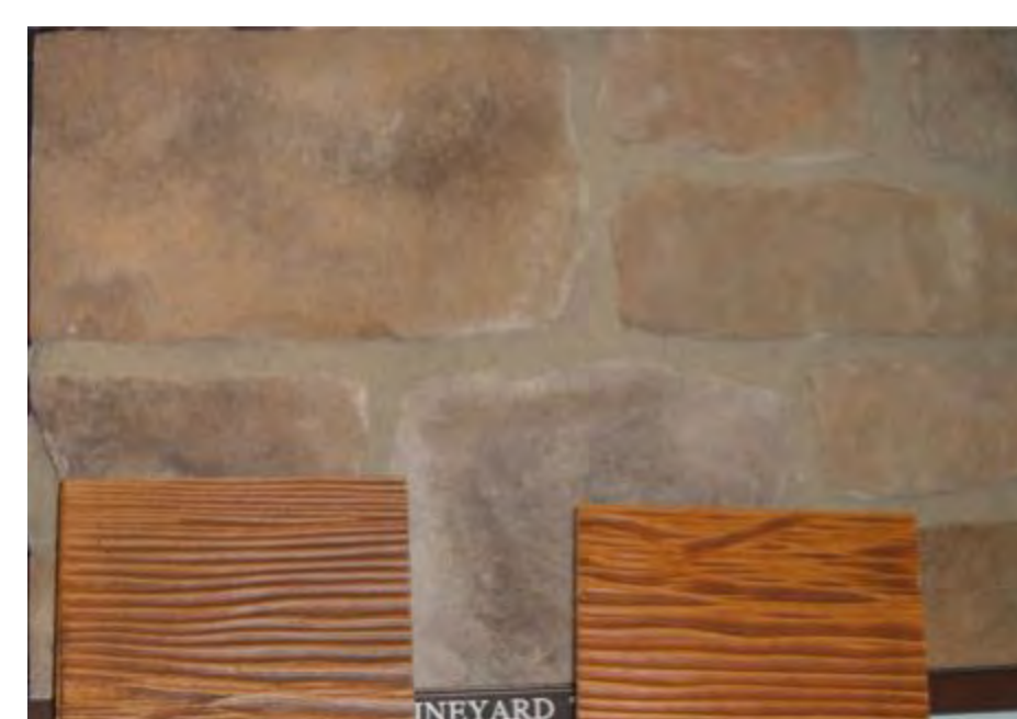
This picture depicts the style of mortar joints that we chose for this project with a different stone.
