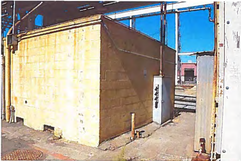
Image 5. South façade, east end. The east façade with electrical vault is visible at the right.
