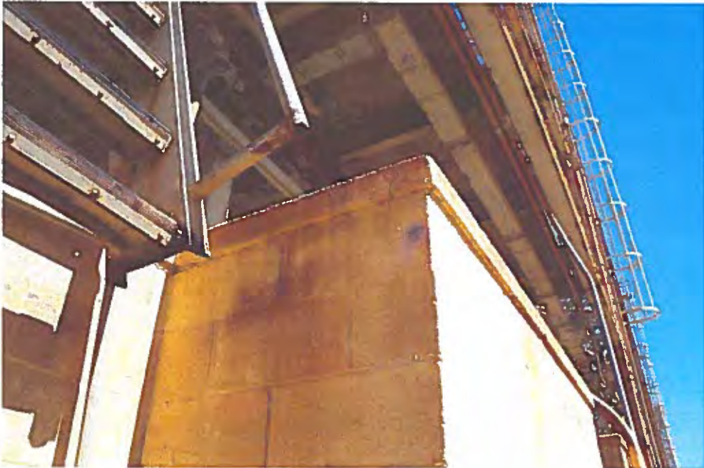
Image 11. Southwest corner, the concrete cap is cracked.
