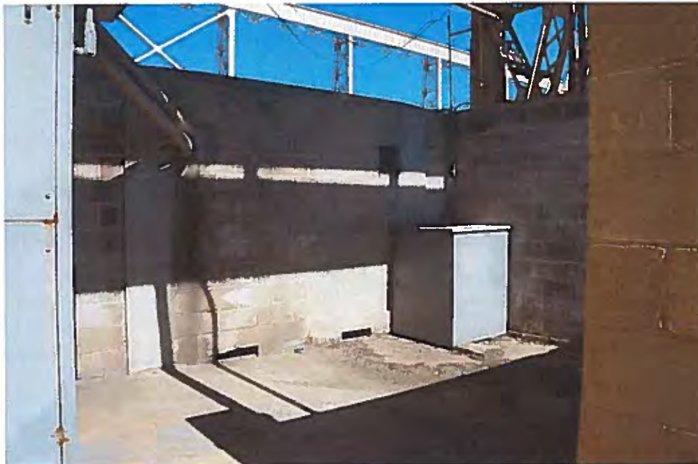
Image 13. Interior view looking north from the south entry. The concrete block walls and floor slab are unpainted. A small electrical vault is visible at the right.
