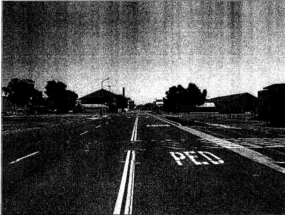
LOOKING SOUTH ALONG RAILROAD AVENUE AT PARCEL "A". EXISTING ROADWAY WIDTH FROM CONCRETE CURB TO AC BERM VARIES 40' TO 24'.
